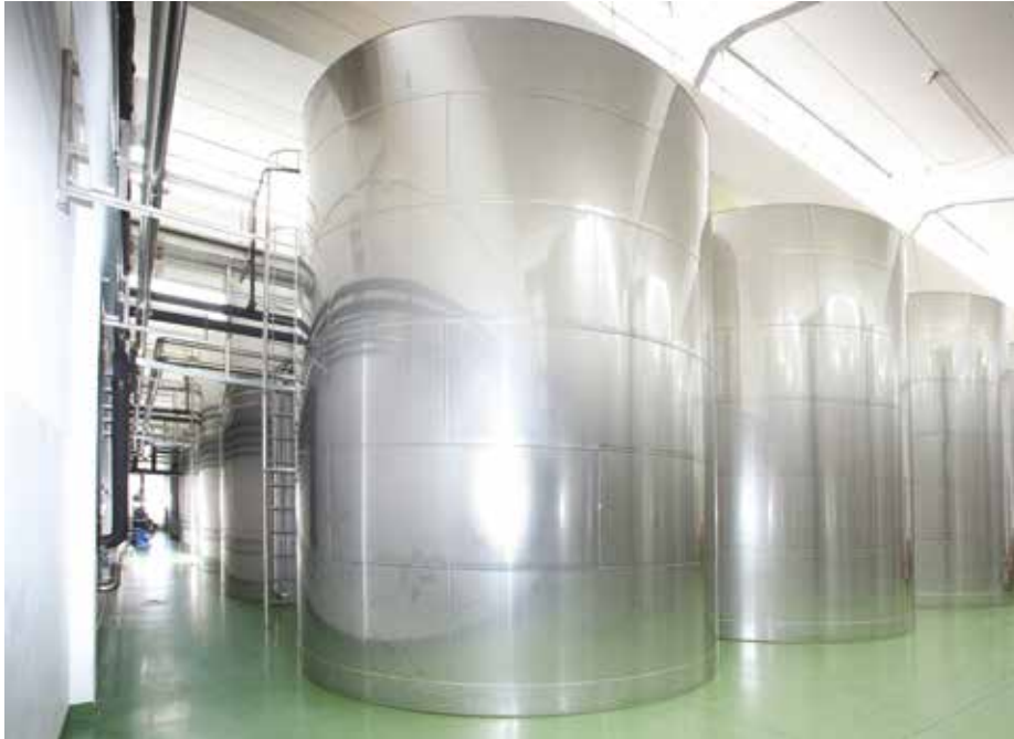
Warehouse B: Insulated Tanks
