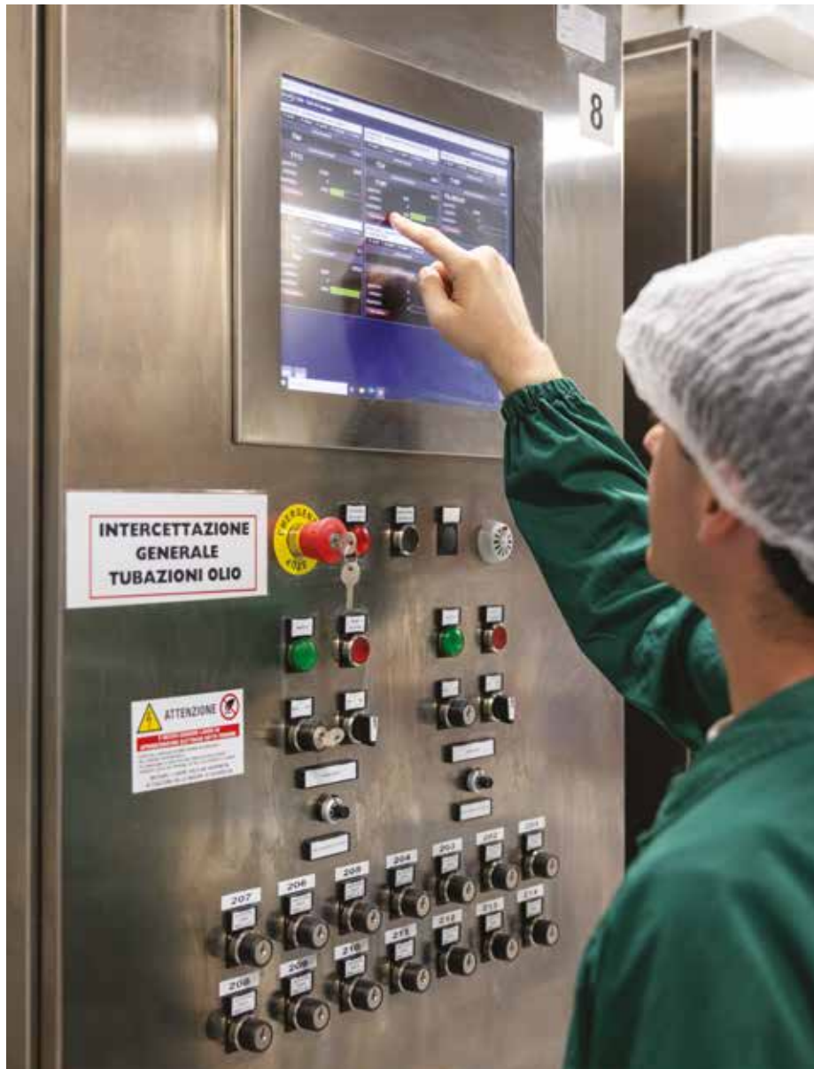
An integrated management and control system for oil discharge, storage and handling of bulk/unbottled oil
